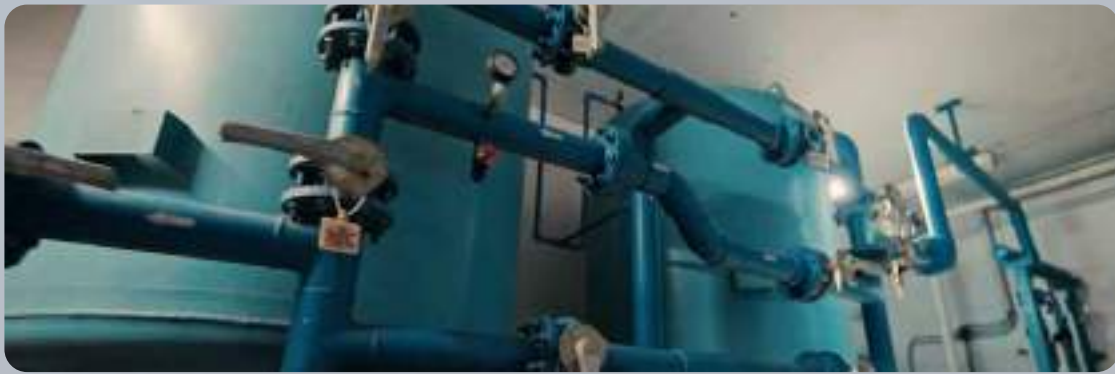
Figure 19. Telkom Group's Sewage Treatment Plant (STP) facilities
