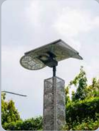
Figure 12. Street lighting with solar PV technology
