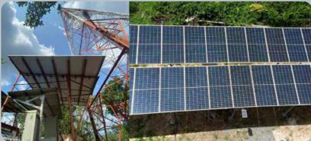
Figure 10. BTS tower with solar PV
