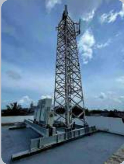
Figure 13. Glass Fiber Reinforced Polymer Tower
