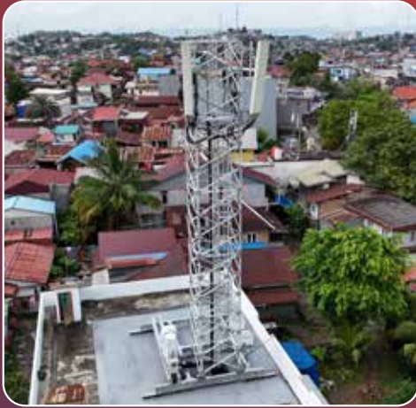
Figure 34. Glass Fiber Reinforced Polymer Tower
